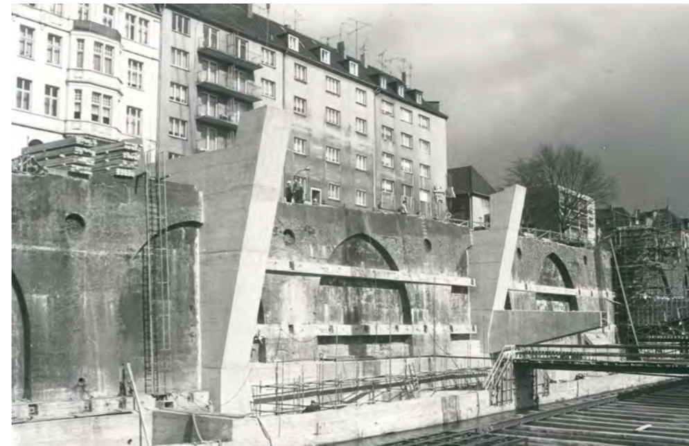
Construction of the supports for the second level of the Altenhagen Bridge on today's Märkischer Ring. Around 1962.
